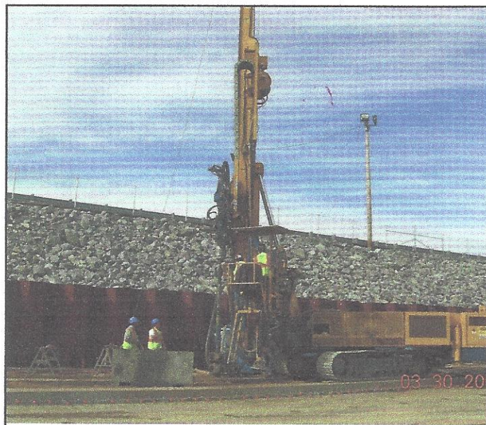
FIGURE 14. LMG Installation Rig used to install casing and remove casing during LMG process (Source: Hayward Baker Inc.)
