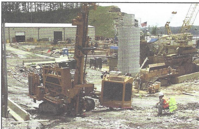
FIGURE 15. Right Rim rock drilling with TSJV cutoff wall slurry and desanding plant in background (Source: Hayward Baker Inc.)
